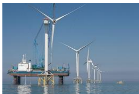
Gambar 3. Ladang angin lepas Pantai ( Offshore wind farm )
